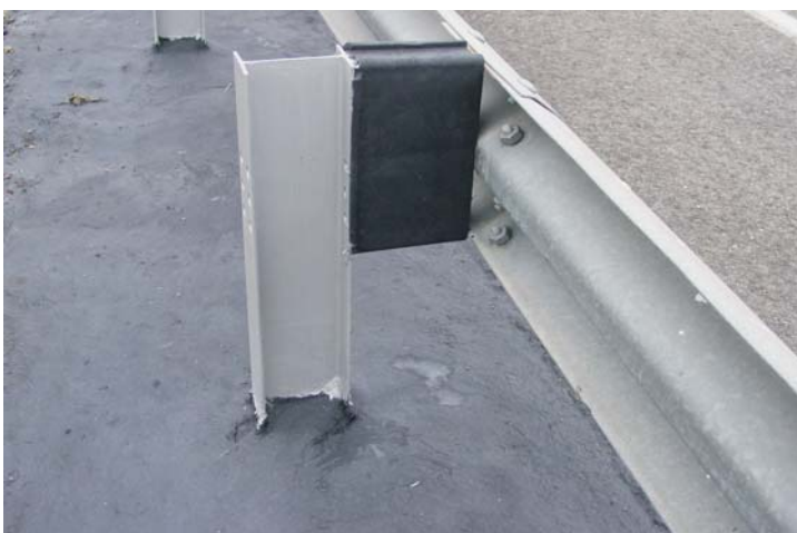
Over spray on the I-Beam posts has been addressed using an aluminum emulsion coating.
