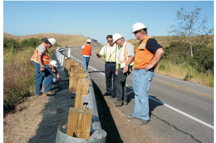
Cal Trans RE, Ray Hopkins (in the foreground), is the on site, daily inspector for this project.
