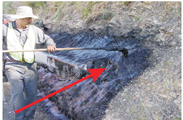
Brushes are used to smooth out composite over this uneven rock surface.
