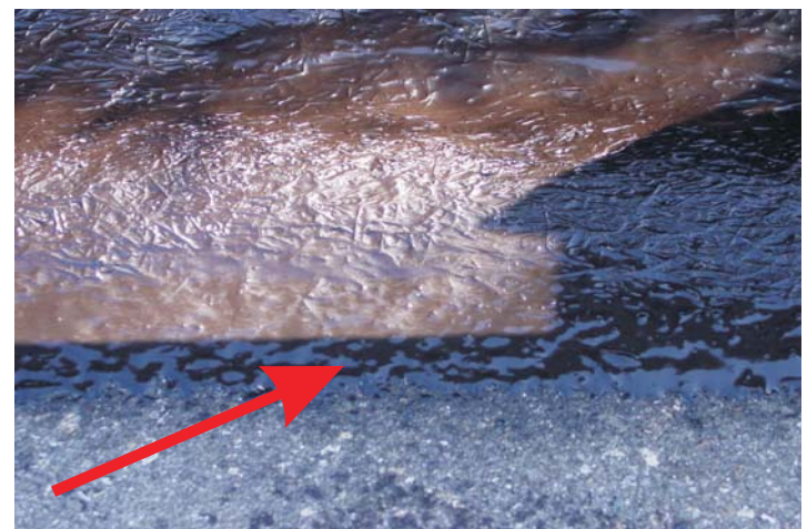
Seamless composite materials also ties into the road AC to prevent water erosion off the road surface.
