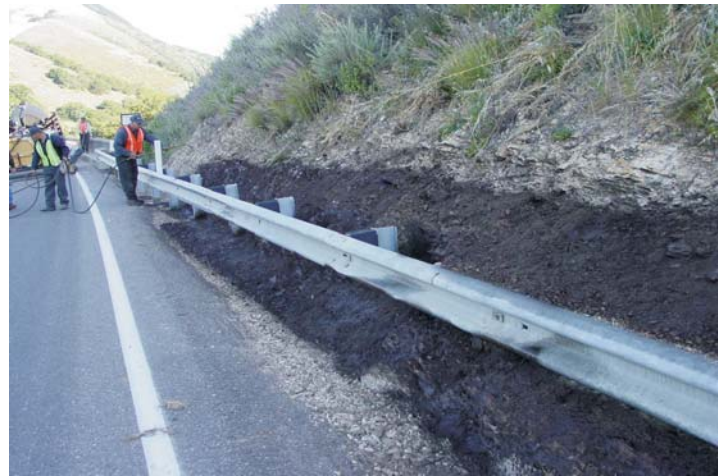
A tack coat of 3-1 121 emulsion and water is then applied to prime the surface.
