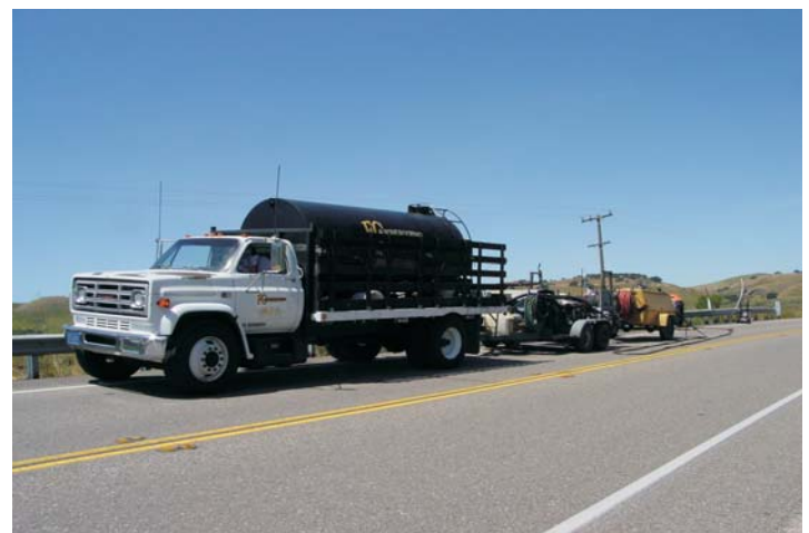
Staged equipment for the installation is a 2,000 gallon agitated emulsion tanker, a Moyno pump, and an Ingersol Rand 185 compressor.
