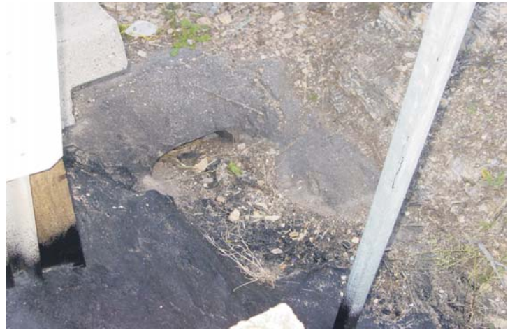
Overside drain will be cleaned out and an application of WeatherWeld will be applied here.
